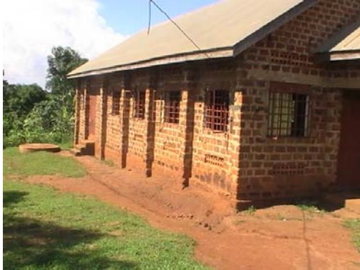
Adventist Church - Base but no tank or guttering
